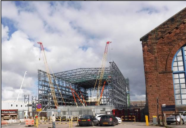
THE CENTRAL YARD FACILITY
